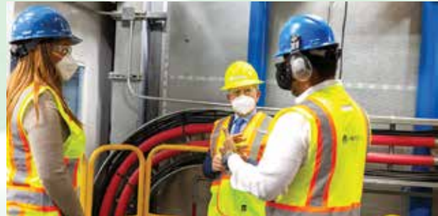
President and CEO Ruth Forbes and Vice President of Engineering, Energy Production and Delivery Don Forsyth discuss the workings of the company's latest generation plant with the Governor.
