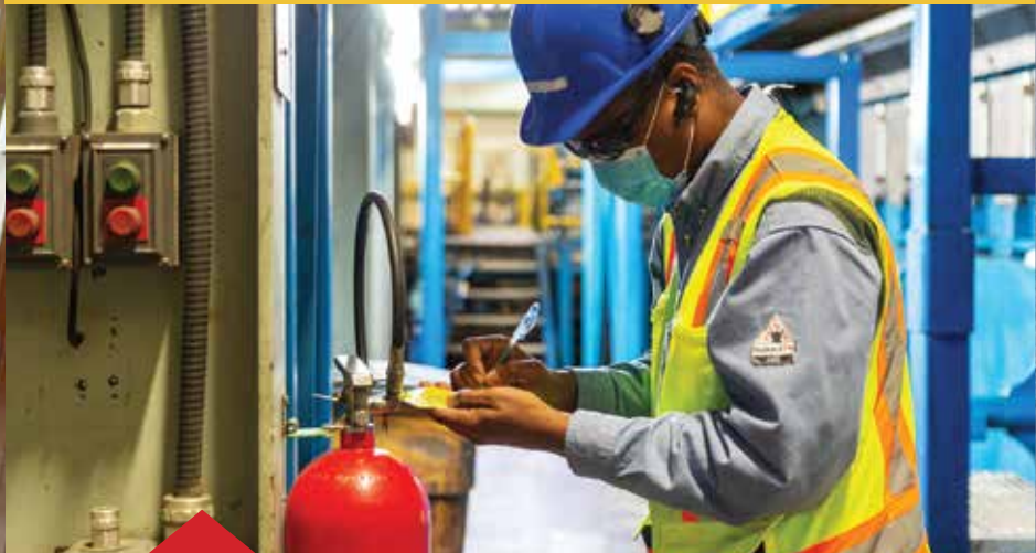
Environment, health and safety matters continued to have priority focus during the pandemic. Here, Senior EHS Coordinator Eustace Musgrove carries out essential inspection of fire equipment.
