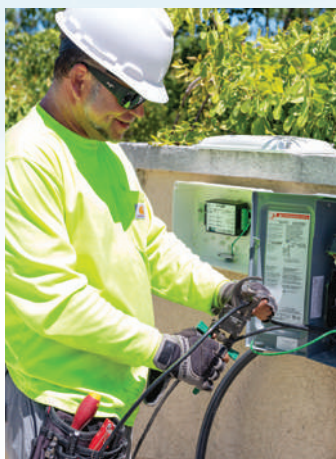
A technician working at the site of a recently installed solar plus battery storage project at a residence in Providenciales. The pilot project launched in August 2019 and will help the company determine the suitability of the technology for its renewable energy programs.
