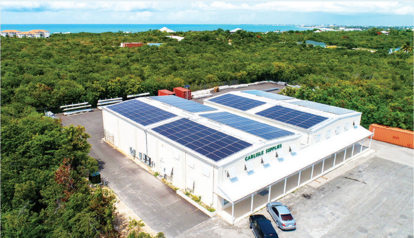
The 105kW rooftop grid-tied solar PV installation at Carlisle Supplies, one of nine participants in the FortisTCI Utility Owned Renewable Energy (UORE) Program.
