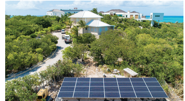
FortisTCI recently launched an integrated solar plus energy storage pilot project at a residential premises in Providenciales. The project will provide data on battery storage usage, costs and technology for the islands.
